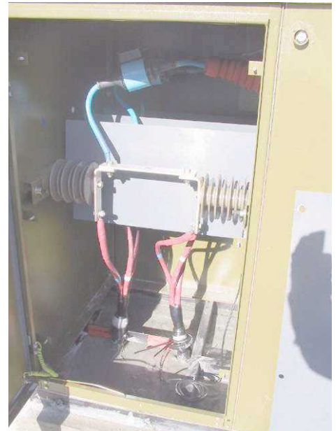
Above right Alstom type Mini-sub HV chamber
